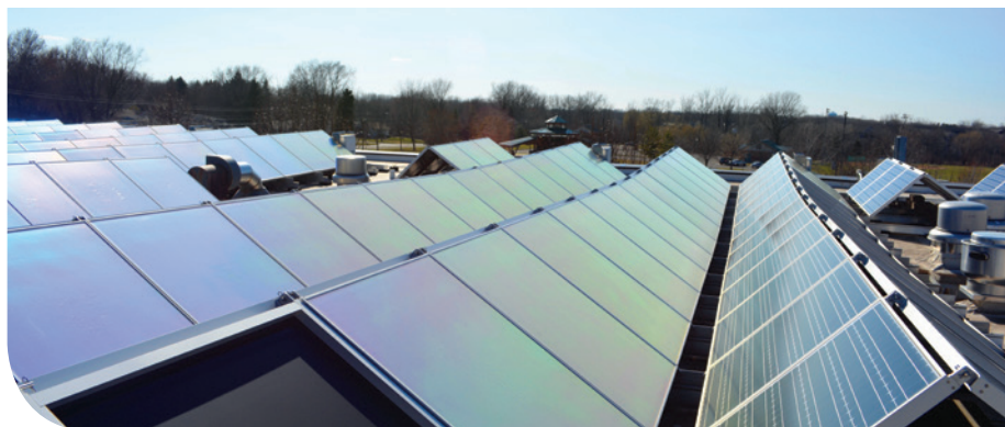
Solar panels were installed on the roof of City Hall in 2012.
